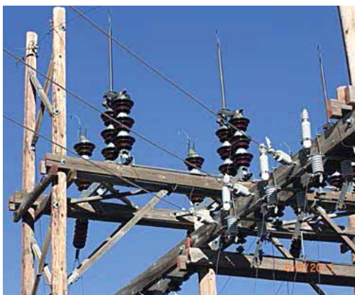
Look closely and you will see a cracked horizontal timber on the left side of the support structure in the South Fork Substation. This substation will be rebuilt in 2013. In the new substation, metal supports will be used.
